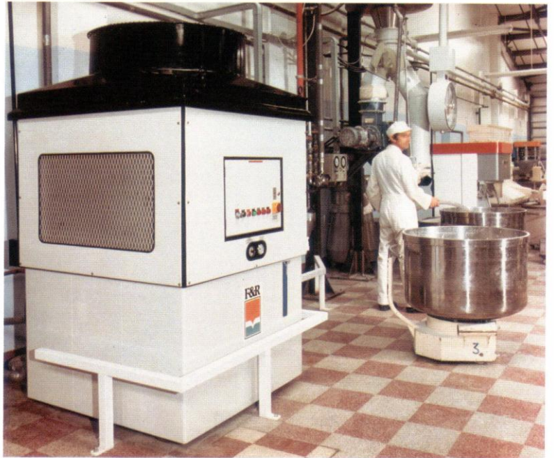
RCU 8-PB supplying chilled water at 1°C to control dough temperature at mixing stage.
